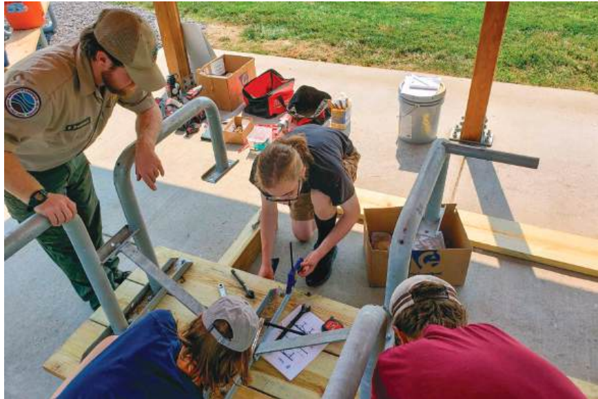
Conservation Corps, a summer project offered by Friends of the North Fork of the Shenandoah River, provided teens with the opportunity to learn more about the environment and engage in community projects, such as the construction of benches and tables at Seven Bends State Park.
